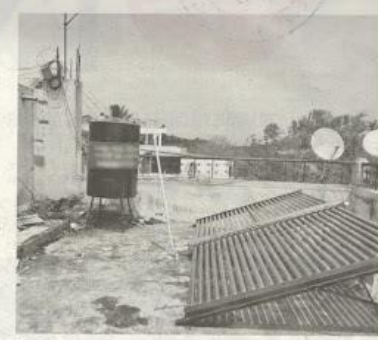
The 3-in-1 boiler of 500 litre designed by Sukanya Dolekar installed at a lodge in Saundatti of Belagavi district | EXPRESS
